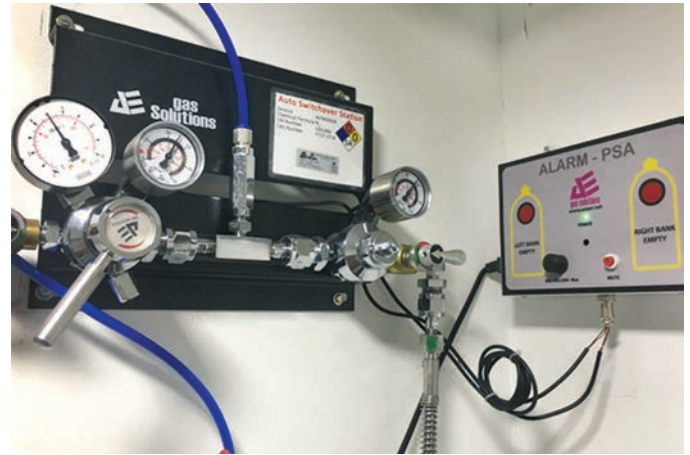
Fig. 5: Monitoring of CO 2 tank pressure with alarm system and autochange for gas cylinders.
